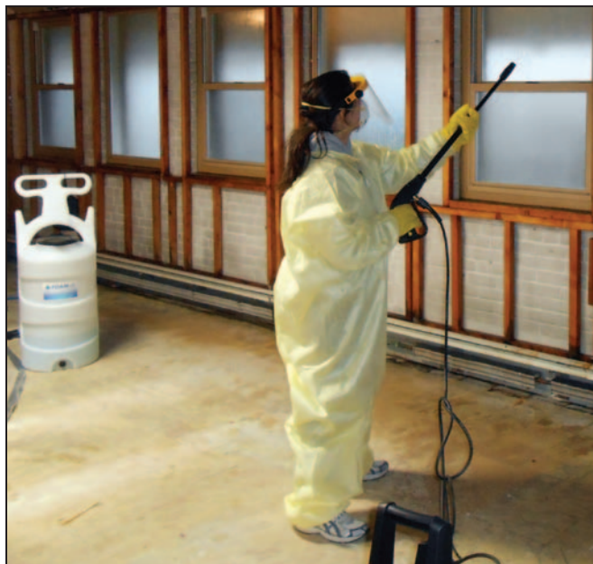
Figure 3. Using a pressure washer to rinse surfaces cleaned with a foam solution
