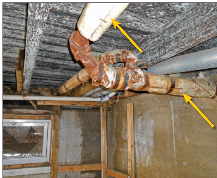
Figure 1: Mold (on wood) and asbestos (yellow arrows) hazard in flooded house
