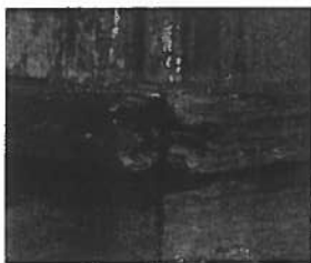
This rotted—and irreplaceable—woodwork...
